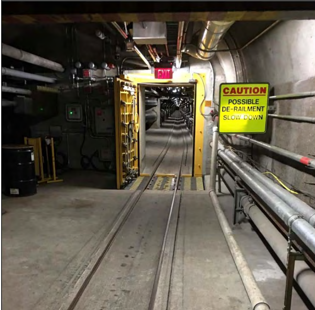
Figure 4.1: Emergency Oil Pressure Door
